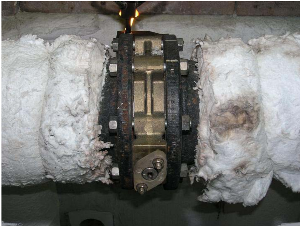
Figure A-2. 8-in. Valve in Furnace After the Fire Test.
