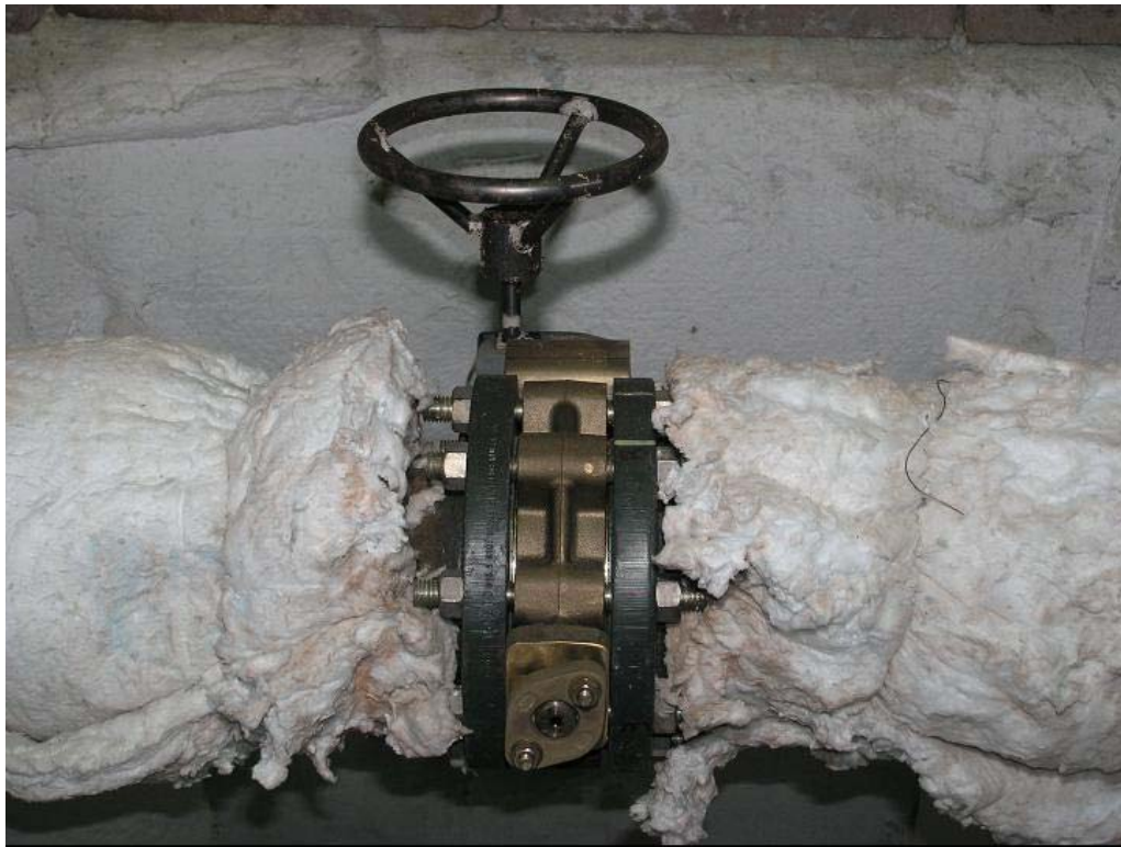
Figure A-4. 4-in. Valve After the Fire Test.
